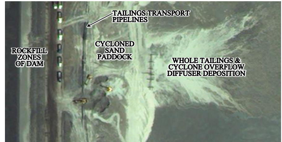
July 16, 2015 WorldView-2 Image of Construction Equipment and Deposition Piping at the Peñasquito TSF- PhotoSat/DigitalGlobe
